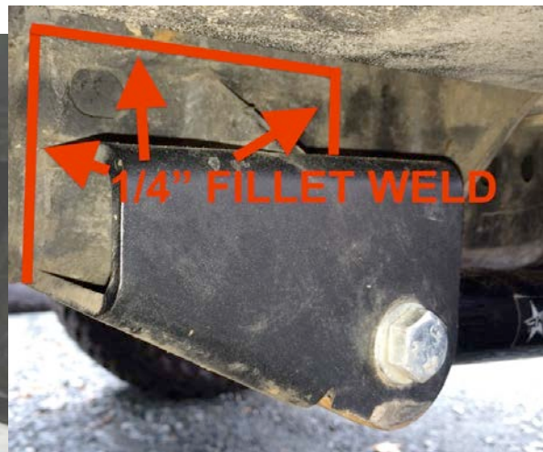
Weld on Lower Control Arm Mount
