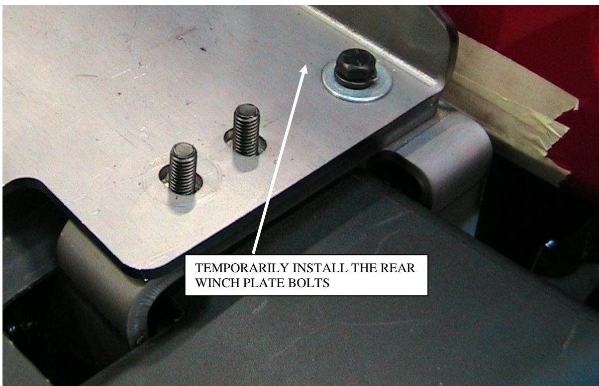
Figure 10: Rear winch plate bolt
