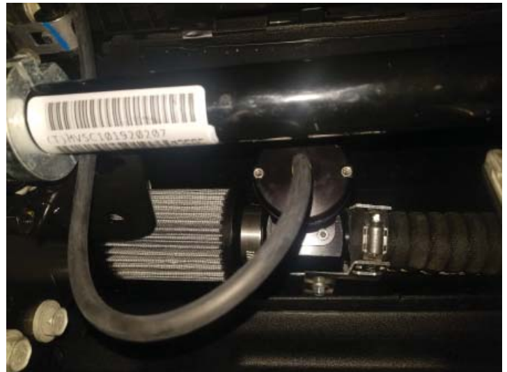
Surge Valve Installed
