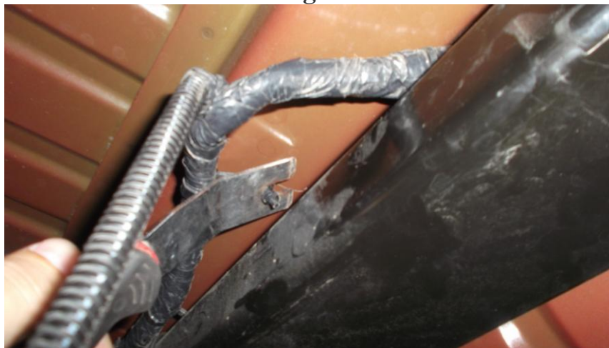
Figure 2. Removing E-Locker Wiring Harness from Cross Member
